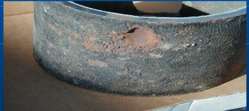
External Pitting of Ductile Iron Pipe in Soil
